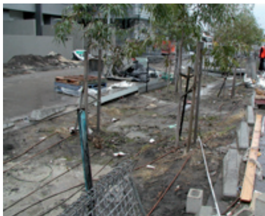
Figure 5. Construction damage is shown with clogging of the bio-retention system surface and loss of vegetation, Victoria Park, South Sydney, NSW.
