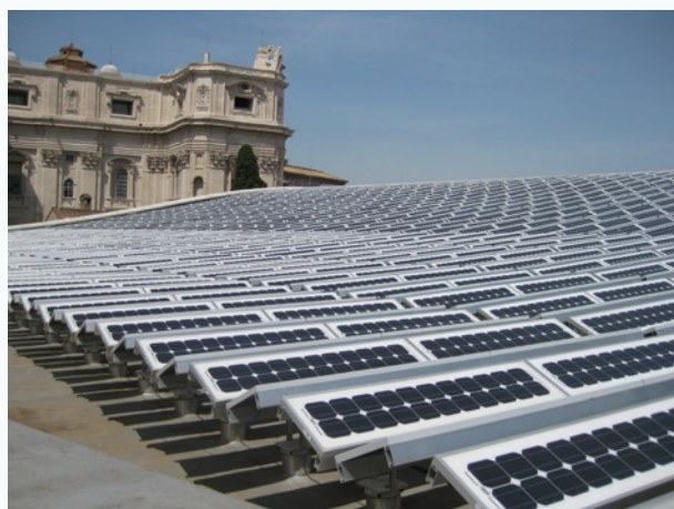
Figure 2: An example of solar PV used in a heritage setting, at the Vatican City. While this might look like BAPV, the PV panels provide an essential shading function to reduce the heat gain of the public papal audience prayer hall and as such are classified as an integrated element of the building construct. (Image: Mats Andersson, Energibanken)
