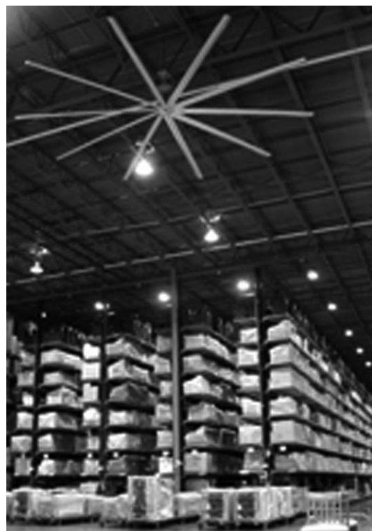
Figure 14. Large HVLS circulating fans in a warehouse
