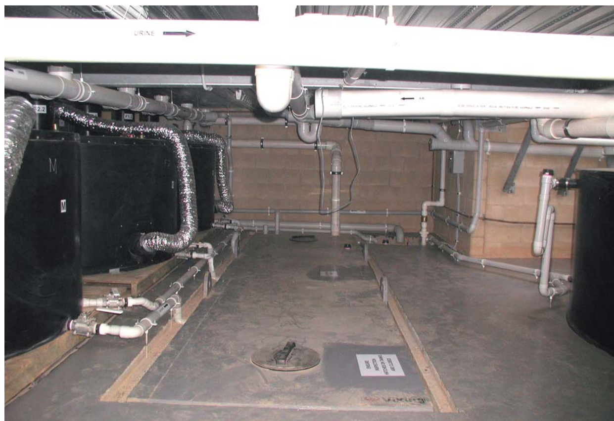
Figure 5 Basement showing composters, in-floor leachate tank and urine tank
