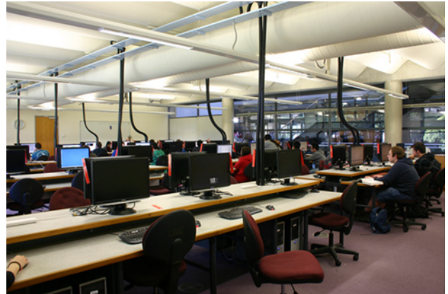
Figure 8 Sine-wave ceiling to computer labs
