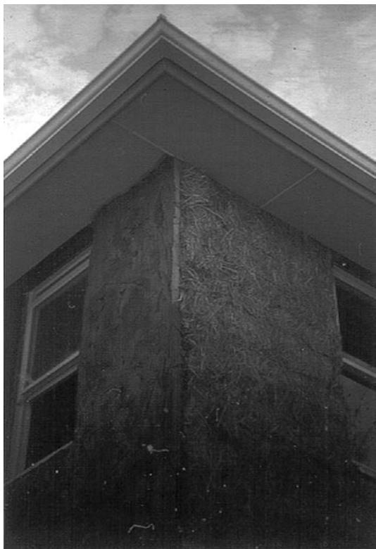
Figure 1. External wall partially rendered to corner
