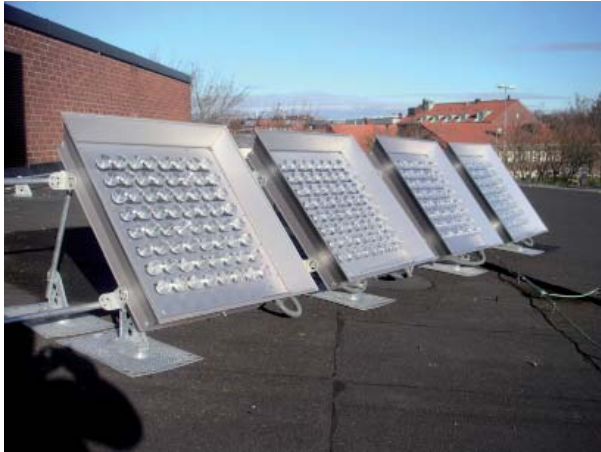
Roof mounted daylight collecting
